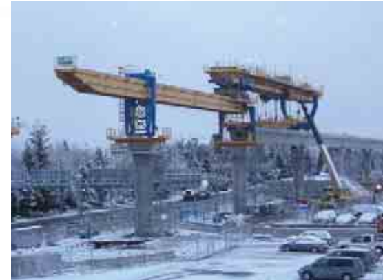
Beams can be assembled in segments on site and put into place using precast segmental construction method.
