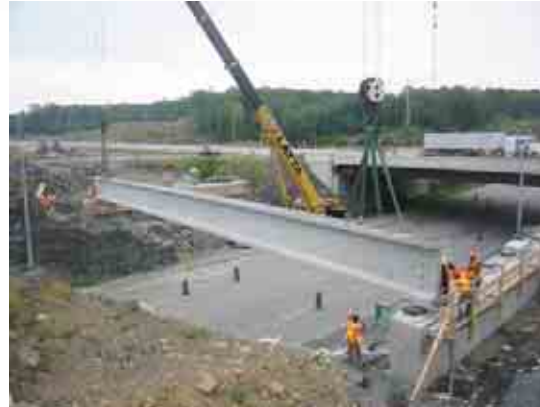
Beams can be transported to the site on a truck and then lifted into place with a crane
