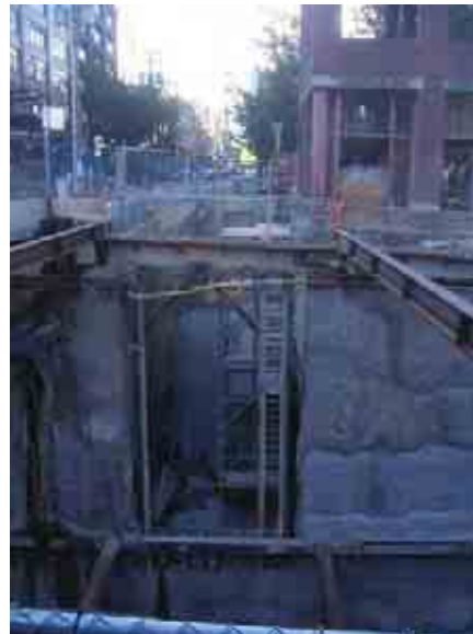
Area is excavated down to track level. To minimize impacts, soil retention systems are used.
